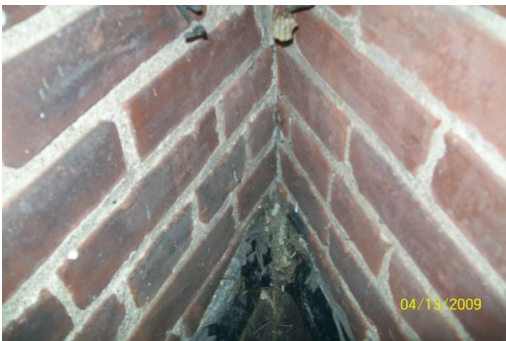
Flashing Failing in Wedge Corner
