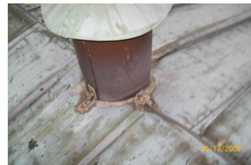
Vent Cracking at roof to base transition
