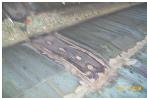
Copper seams failing (typical)
