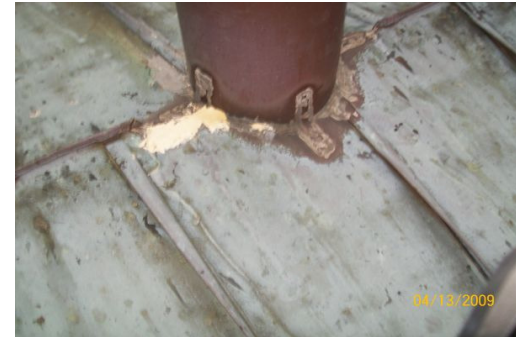
Vent Cracking at roof to base transition
