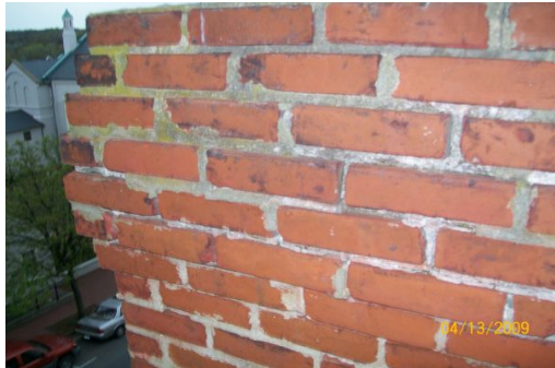
Chimney Masonry Failing (typical)
